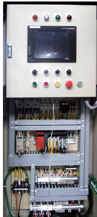
Control devices (Control panel)
